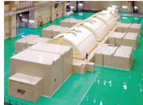
Nuclear Power Steam Turbine Generator
