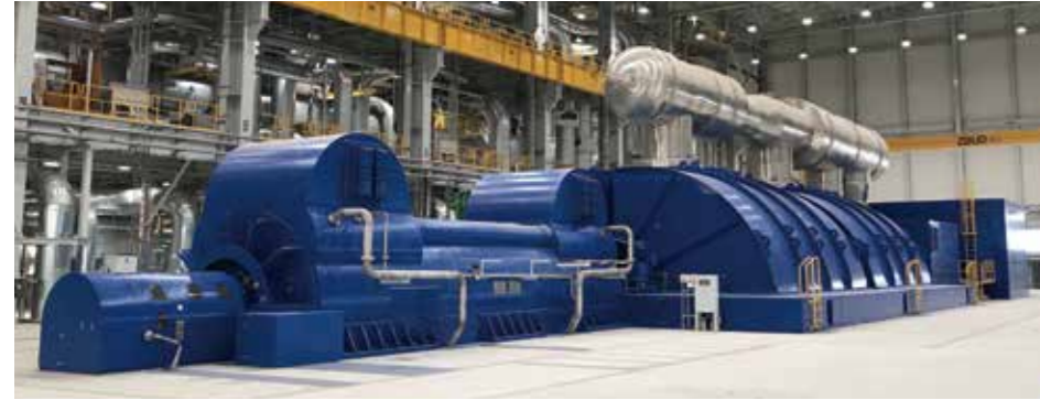
Thermal Power Steam Turbine Generator
