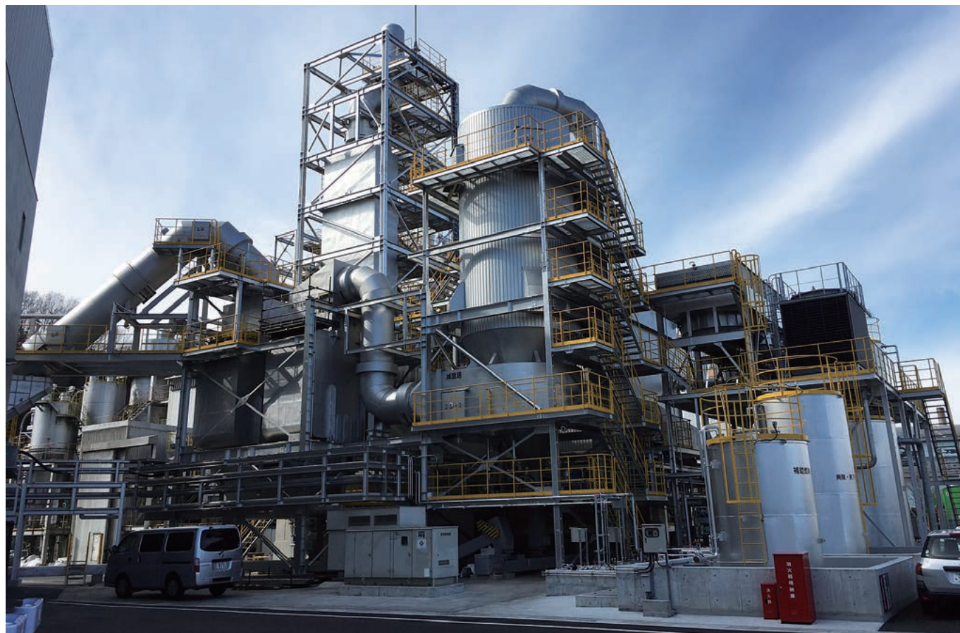
産廃焼却施設 / Industrial waste incineration facility
