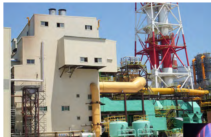
BFG/COG/NG焚ボイラ(350t/h) BFG/COG/NG firing boiler(350t/h)
