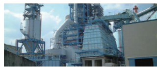
循環流動層ボイラ (CFB: Circulating Fluidized Bed)
