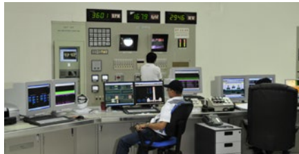
Pagbilao Control Room
