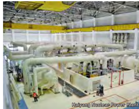
Nuclear Power Turbine Generation Equipment
