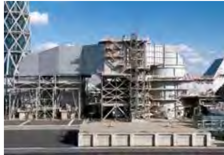
FGD (Flue Gas Desulfurization Plant for Coal-Fired Boiler [1,000 MW]) Wet Limestone-Gypsum Process
