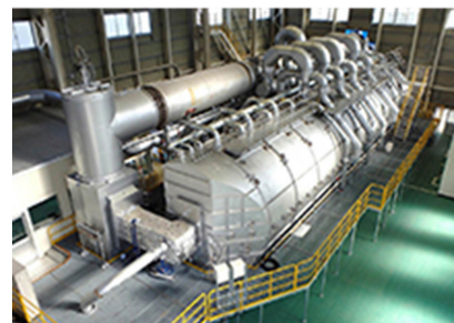
Figure 2 Example of large combustion test equipment (Operation started in 2014)
