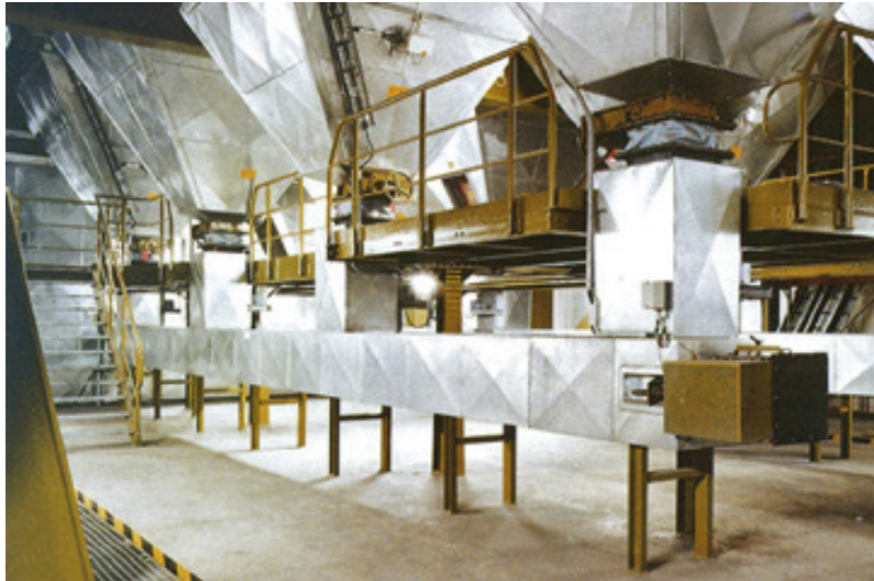
Ash removal system for large steam generator
