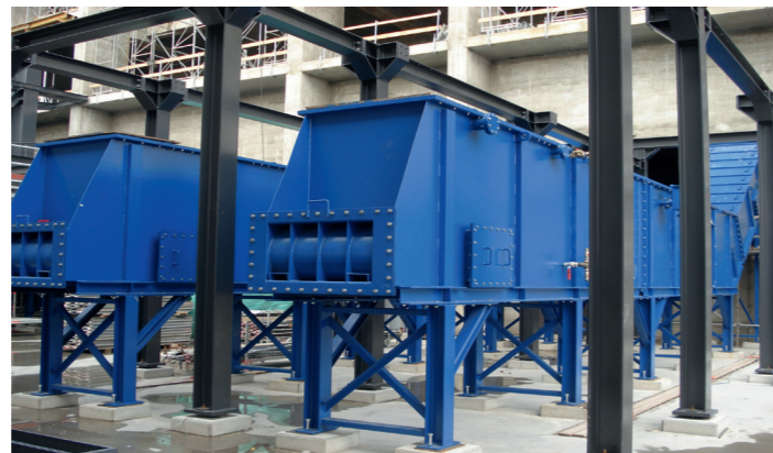
Submerged apron ash conveyor
